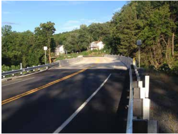
This bridge spans the Maiden and Saucony creeks on Route 143 between Richmond and Perry townships. Constructed in 2010, it replaced a bridge that had been closed since 1998.
