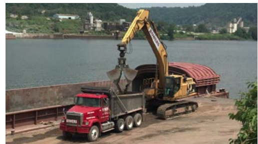
Flyash transfer from barge to truck
